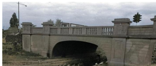
Figure 8 Bridge before 2003 "Upgrade"
